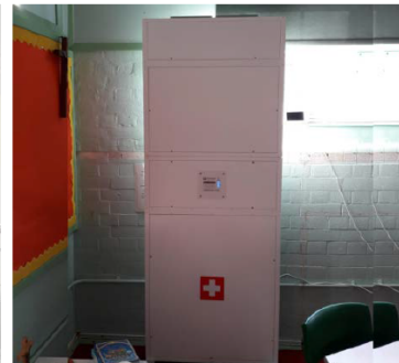
Air purifier in classroom at St Mary's
