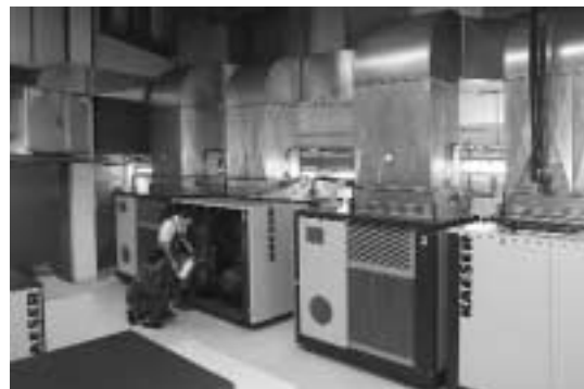
Figure 5 - Maintenance of a compressed air system at Porsche (Copyright Druckluft Effizient)
