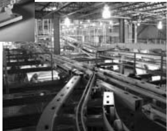
Baggage handling at Charles de Gaulle Airport (Copyright Siemens)
