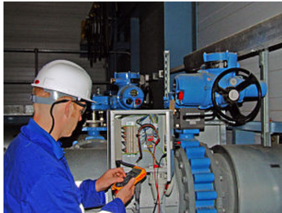
Figure 11 – An electrical actuator on a valve in a power plant (Wikipedia, by Khepster, published under the Creative Commons Attribution 3.0 License ).
