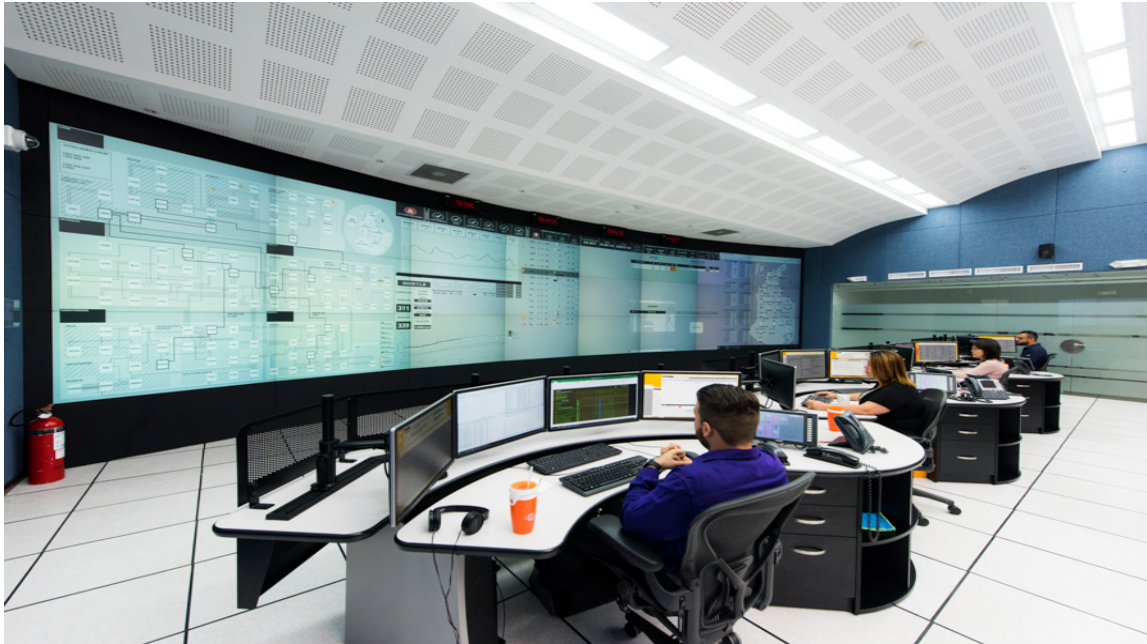
Modern control centre, 2019 [Courtesy of XM Colombia] Challenges: inaccurate forecasting, control of large number of gens, new transmission operation criteria, security risks, changing flow patterns, etc.
