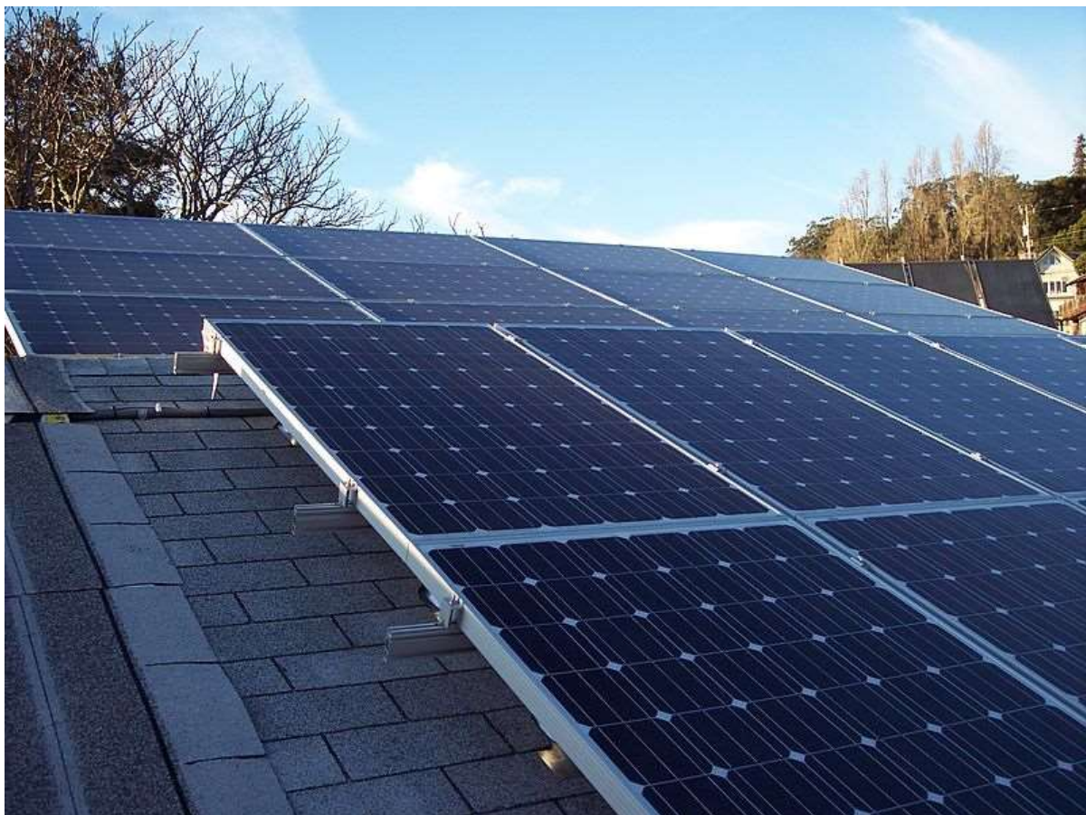
FIGURE 1 – ROOF-MOUNTED PHOTOVOLTAIC SOLAR MODULES AT 2415 PROSPECT STREET IN BERKELEY, CA, USA (PHOTO: ALFRED TWU, LICENSED UNDER CREATIVE COMMONS CCO 1.0)
